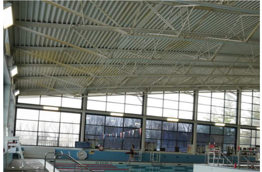
Discoloration of painted steel metal decking
