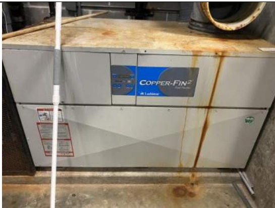
Figure 23 Lochinvar pool heater (corrosion)
