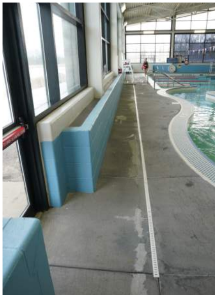
Cracks in colored concrete pool deck
