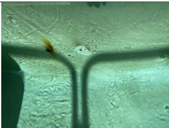
Figure 9 Rebar bleed through
