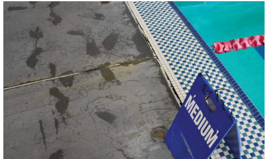
Failing expansion joint caulking
