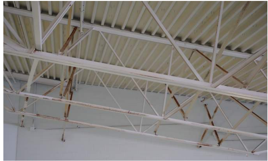
Rust on steel roof trusses
