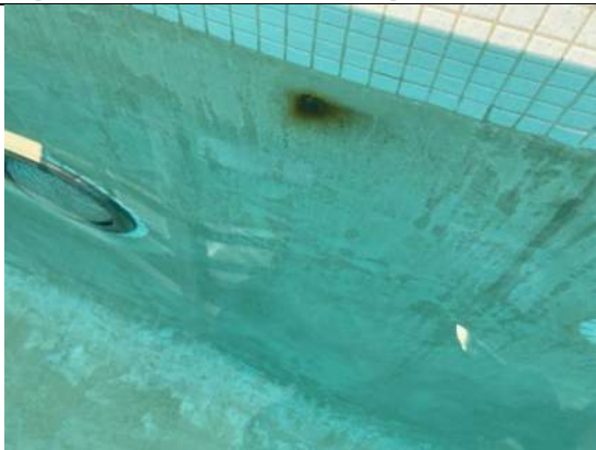
Figure 11 Rebar bleed through
