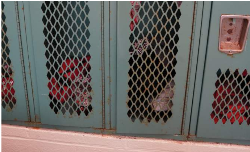
Prefinished metal locker with signs of rusting
