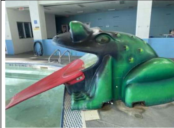
Figure 13 Frog Slide (Corrosion at base)
