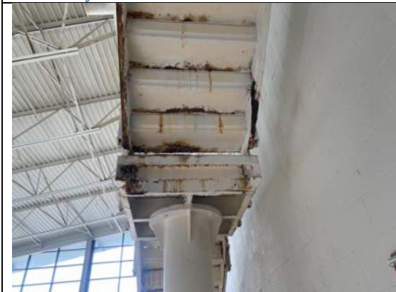
Figure 17 Waterslide tower corrosion
