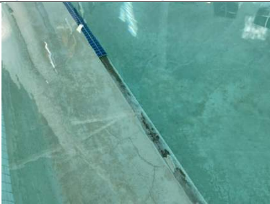
Figure 12 Missing tile on underwater bench
