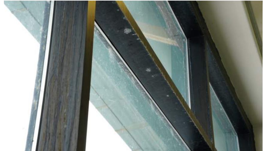
Minor staining of anodized aluminum frame system
