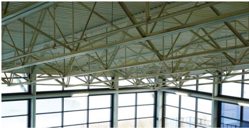
Discoloration on steel roof trusses and metal decking
