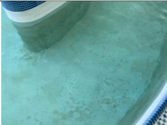
Figure 7 Plaster staining and discoloration
