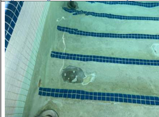
Figure 15 Plaster spalling and delamination on stair entry
