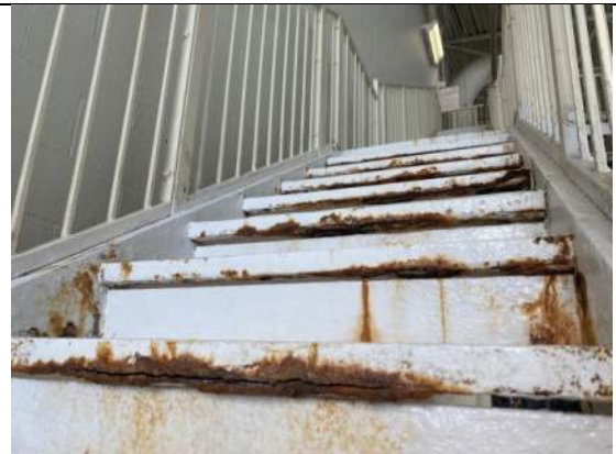
Figure 18 Waterslide tower stair corrosion
