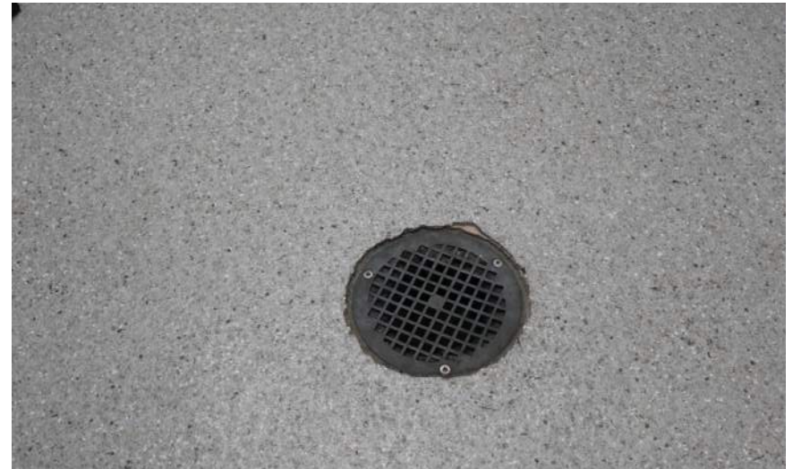
Slip resistant vinyl floor at floor drain
