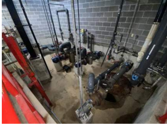
Figure 20 Recirculation pump pit
