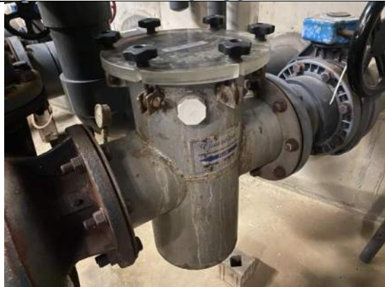
Figure 22 Recirculation system components corrosion
