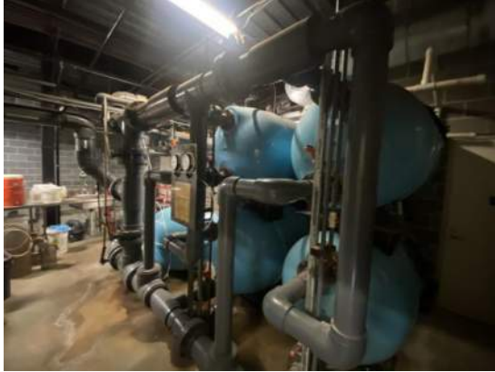
Figure 19 High-rate sand filtration
