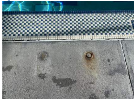
Figure 16 Corrosion on deck anchors
